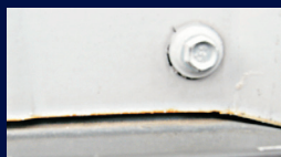
Environmental tests show extensive corrosion along the cut end of a panel without Edge-Rust Inhibitor.
