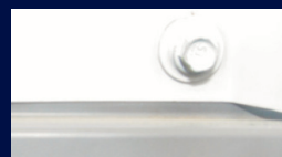
Minimal corrosion is detected along the cut end of a panel with Edge-Rust Inhibitor application.
